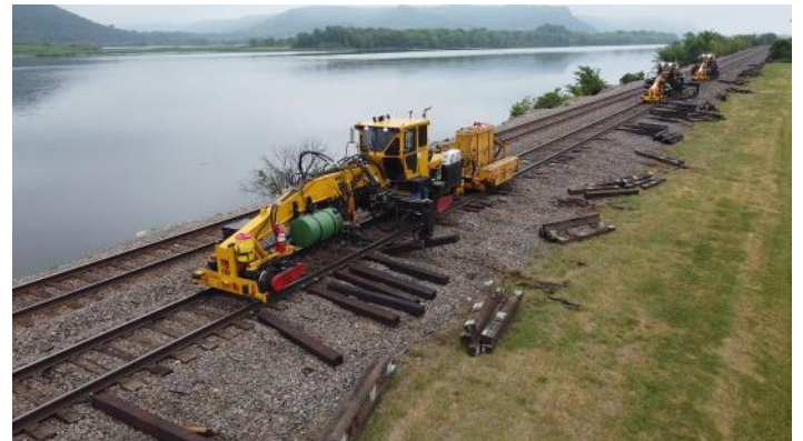
Nordco tie inserters (three of them) slide new ties into the empty cribs. For speed and efficiency, there are multiple machines of the same type handling each task: the first one moves far ahead and works a certain number of ties, the second works a like number, and the third handles the remaining ties. If a machine were to develop a problem, there are a couple others nearby so production can continue, albeit at a reduced rate.
