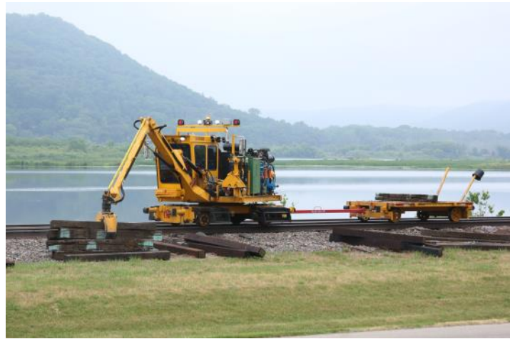
Another tie crane places new ties on the ballast shoulder adjacent to the empty crib. Note the ties piled up in front of the machine - they are pushed along the top of the rail to be used ahead. If there are more ties than cribs, the excess are placed on the trailer dragged behind the tie crane. Likewise, if an operator runs out of ties, a few can be taken from this reserve.
