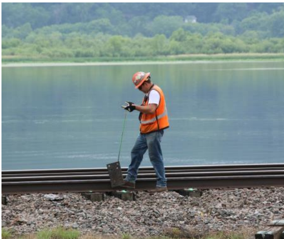
Workers pick up the tie plates and manually place them on the tie ends.
