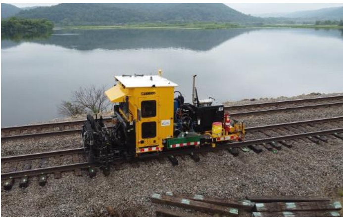
The tie plate inserter raises the rails and slides the tie plates into position, and lowers the rails onto the tie plates. Racine Railroad Products developed its first tie plate inserters in the early 2000s; this, the Advanced Tie Plate Inserter (ATPI) was introduced in 2017.
