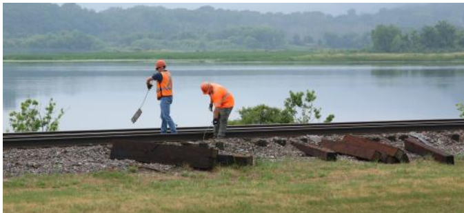
A couple workers equipped with long hooked rods manually remove the tie plates. These will be reused when the new ties are inserted.
