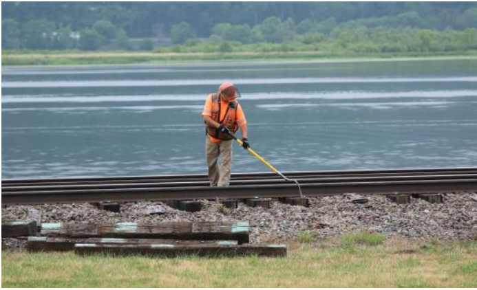
A worker manually removes any remaining ballast. This final cleaning step is important because the tie plate (next step) needs to rest on a clean tie surface.
