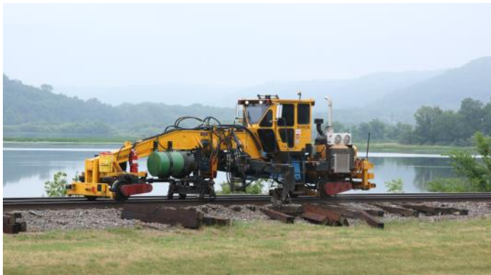
The second tie remover pulls the old tie out completely. The empty space left by the tie is known as a crib. This equipment was manufactured by Nordco, of Oak Creek, Wisconsin.
