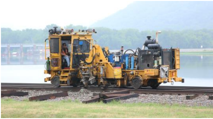
The first tie remover pulls the old ties partway out from beneath the rail. In this step, the rails are lifted so the tie (and tie plate) may be easily slid out. The bulging pile of ballast hints at the amount of force this machine exerts on the tie.
